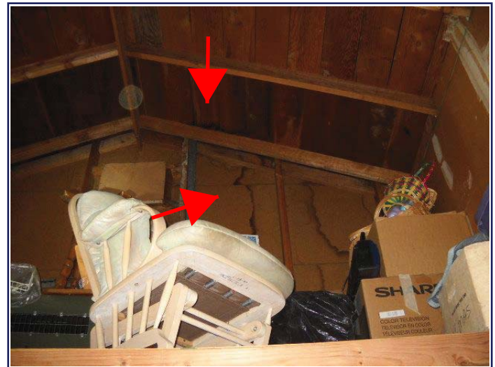
Stains visible at the left side of the garage.
