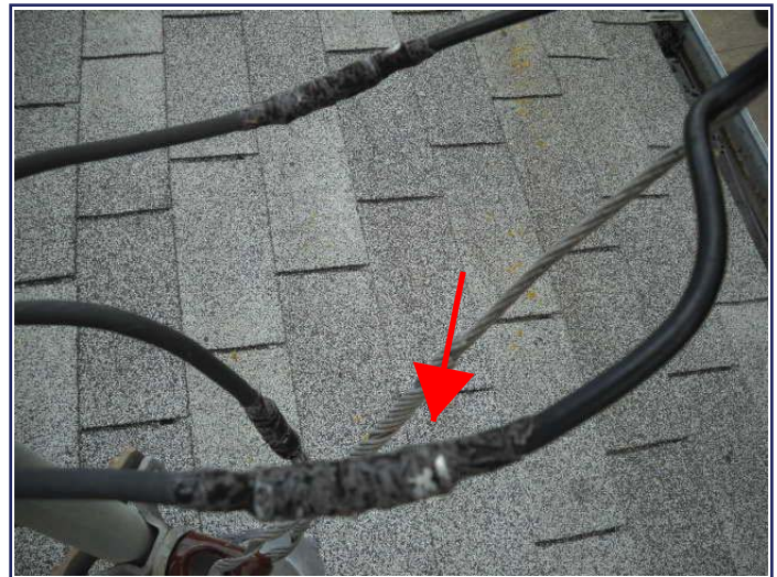
Deteriorated insulation at the electrical service drop wires.
