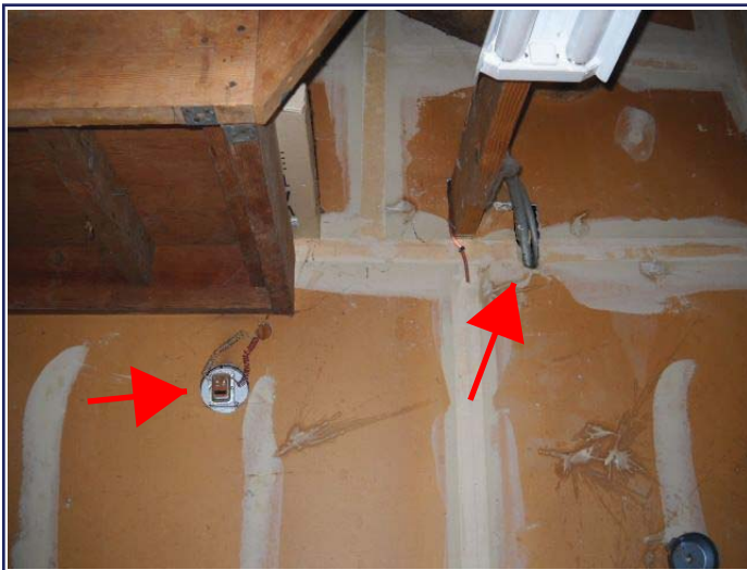
Some of the unsealed firewall penetrations at the right side of the garage.
