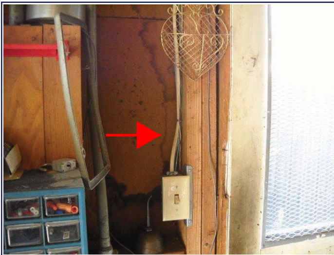
Unprotected wiring below 7ft in the garage.
