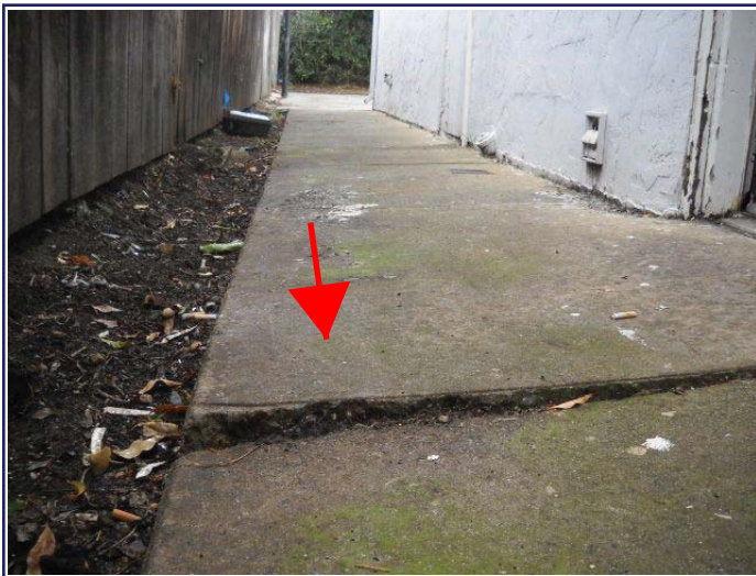
Trip hazard at the left side walkway.
