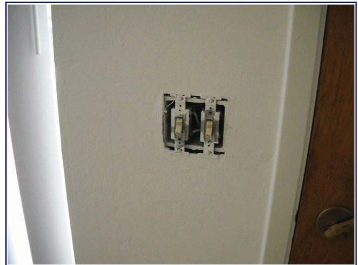
Missing switch cover plate in the living room.
