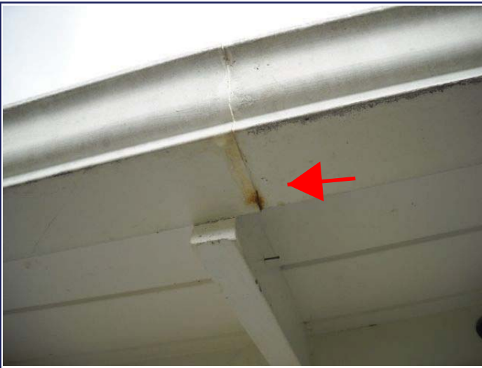
Leaking gutter joint.
