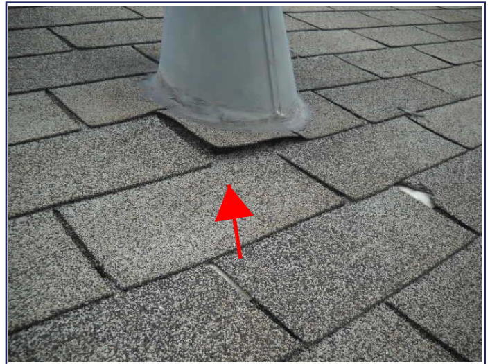
Lifted shingle at the front roof.
