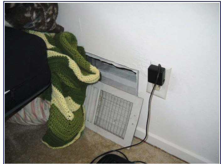
Loose heat register cover in the front bedroom.
