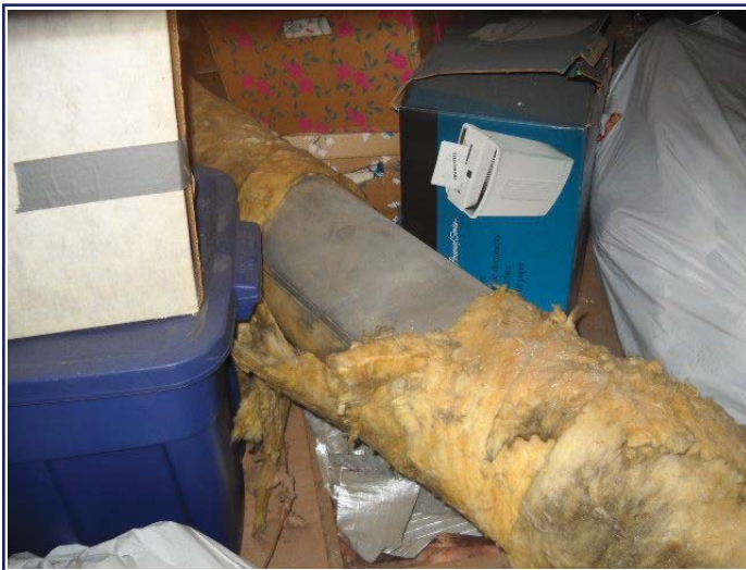
Torn and missing duct insulation in the attic.
