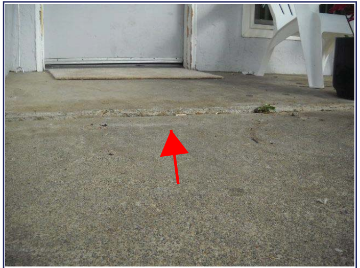
Trip hazard at the front of the house.
