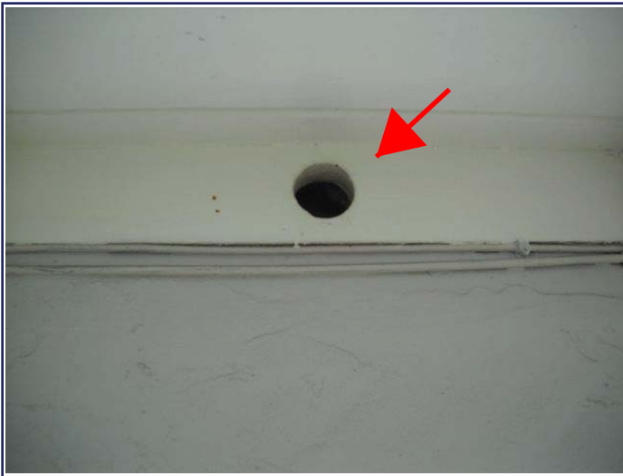
Missing garage vent screen at the front of the house.
