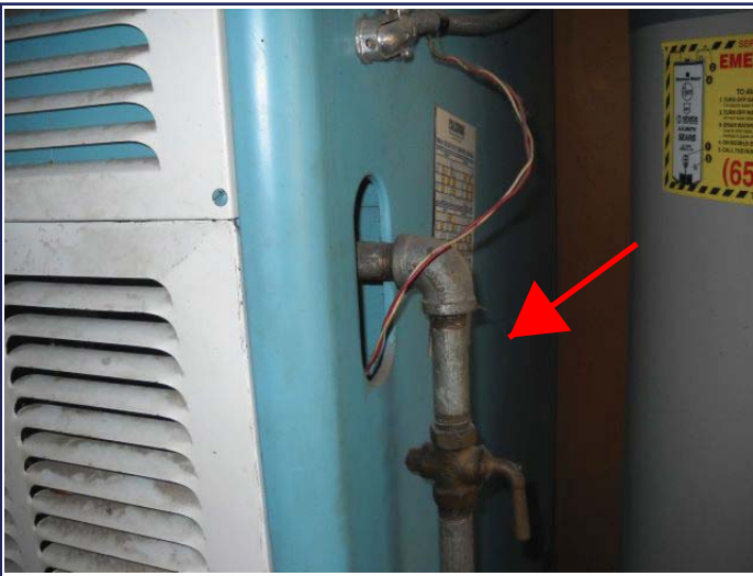
No flexible connector at the furnace gas supply line.
