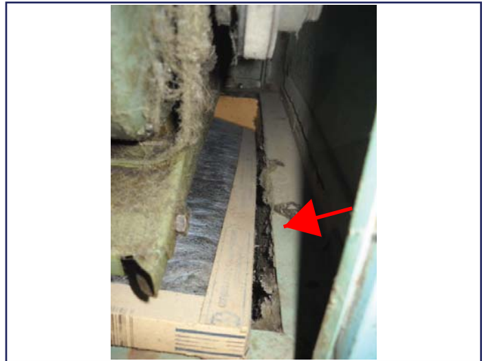
Undersized return air filter inside the furnace.
