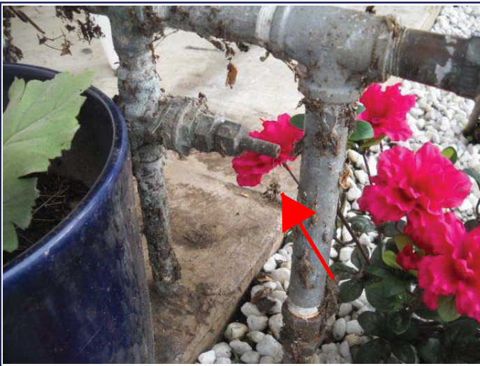
Missing handle at the main water shutoff valve.
